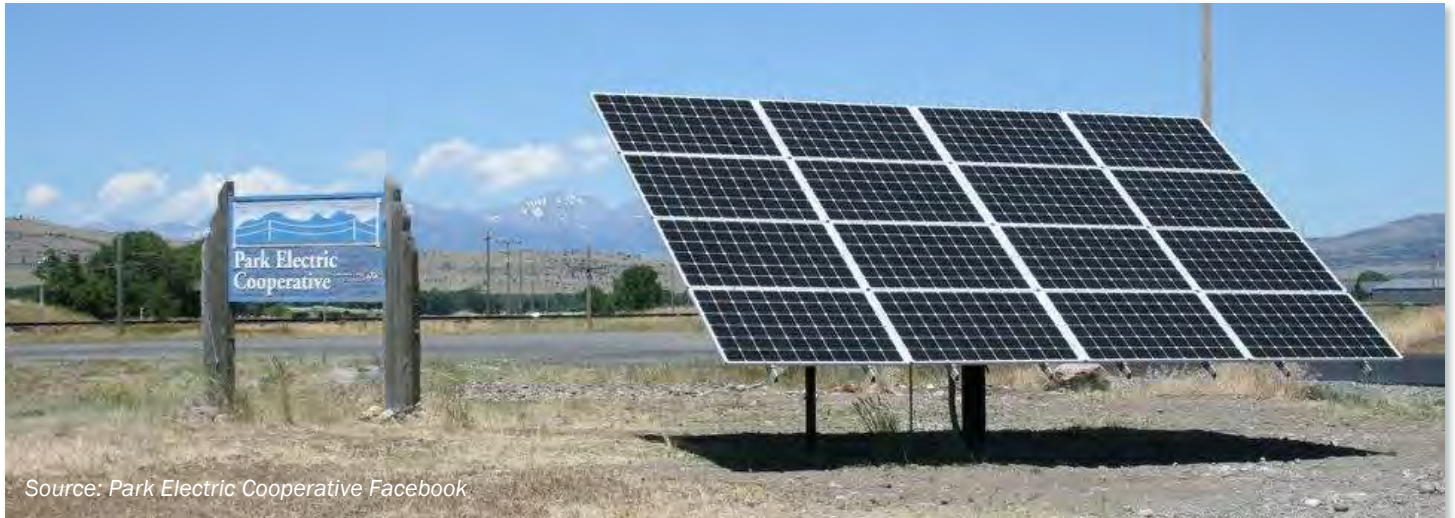
Figure 9.1: Park Electric Cooperative
